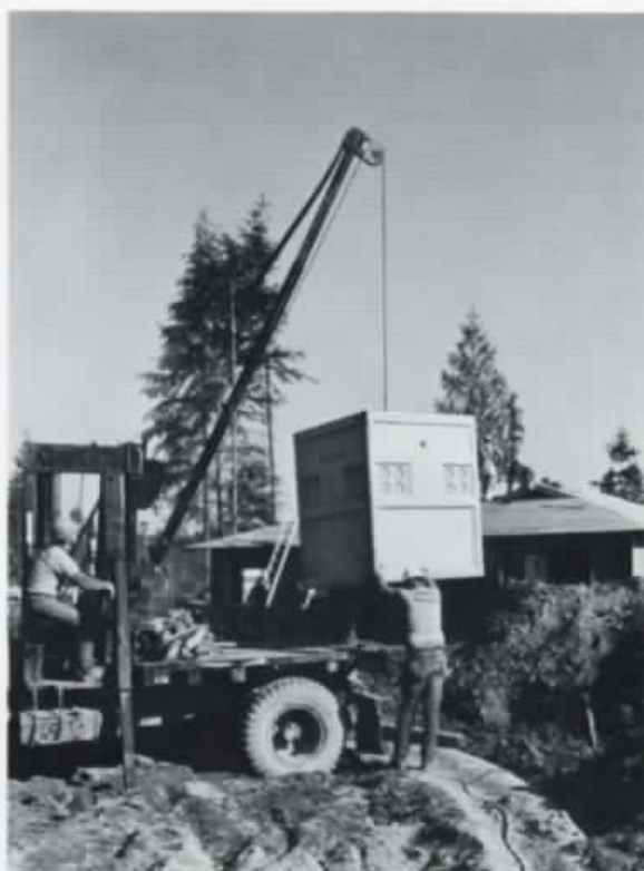
Asplundh Service Company crews expanded into other areas of underground and overhead distribution construction.
